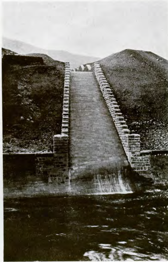
Discharge Chute Yeoman Hey Bye-pass
