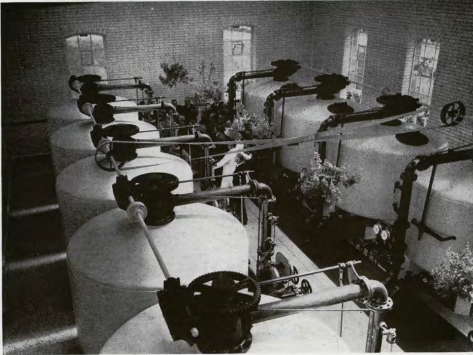
10 New Pressure Filters at Ashway Gap
