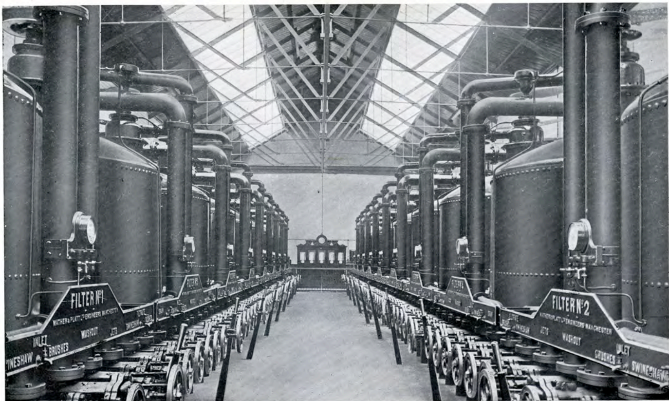
BRUSHES FILTER HOUSE
