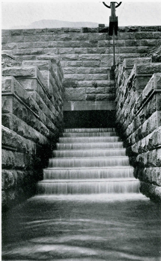
Outlet from pool below primary leaping weir at Yeoman Hey embankment. The secondary leaping weir is situated immediately below, and it is possible to discharge the water flowing from the pool either into Yeoman Hey reservoir or into a conduit connected to the filter house.
